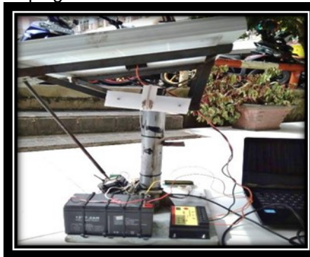
Gambar 4.3 Tampak Samping Panel
